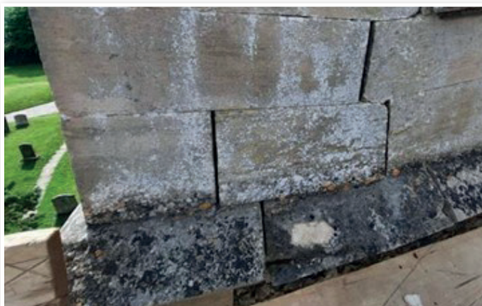
Hollow and insecure stones section found during inspection
