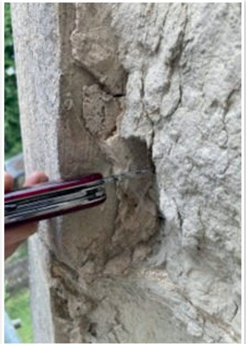
Tottenhoe Clunch stone is friable and in poor condition in several areas inspected
